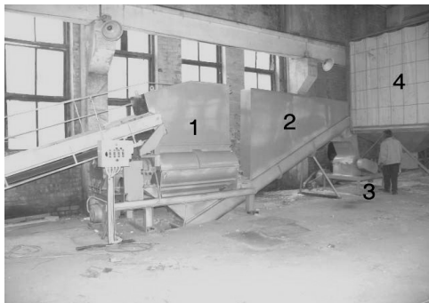
Fig. 11. Crushing line for waste EPS packages:
