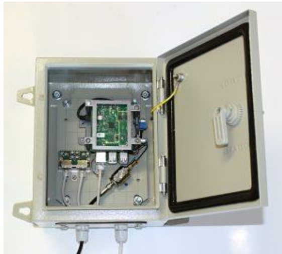
Figure 51. LoRaWAN gateway equipment used for experiments.
